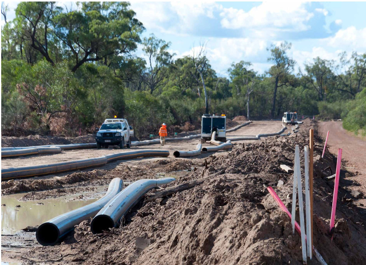
The laying of coal seam gas pipes across bushland in Tara, Queensland. Image: Jeremy Buckingham.
